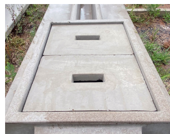
Float Valve Chamber with Split Lid
