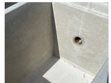
Float Valve Chamber
