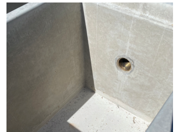
Float Valve Chamber
