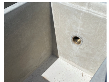
Float Valve Chamber
